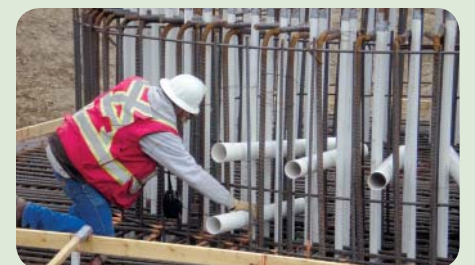
Assembling the rebar as part of the concrete foundation for a wind turbine. The foundation will eventually reside below the ground.
