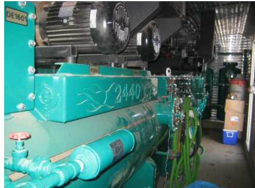
DPVE treatment system in Lions Park.
